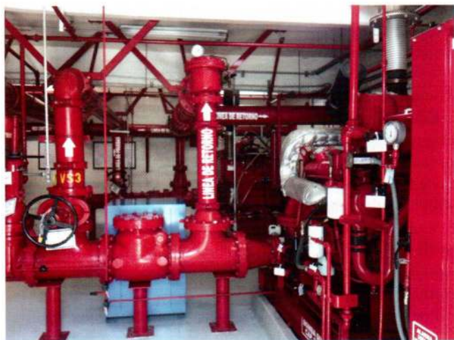
Space use for two fire protection pumps.
