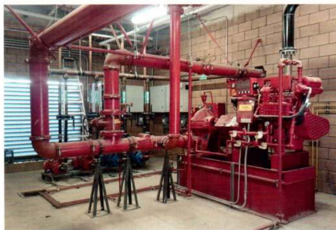
Space for one fire protection pump in a room that was designed for two fire pumps.
